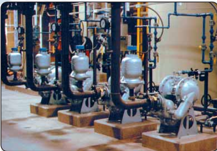
HDB bottom discharge ported pumps with tranquilizers installed at an industrial waste treatment facility.
