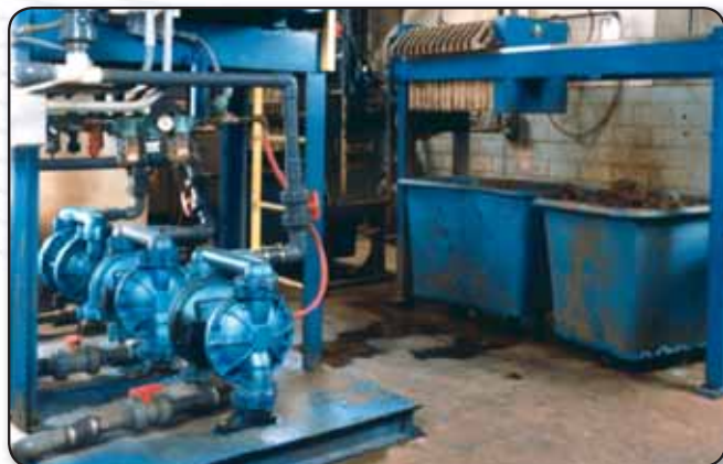
Metallic standard duty pumps handling suspended solids in an industrial waste treatment operation.
