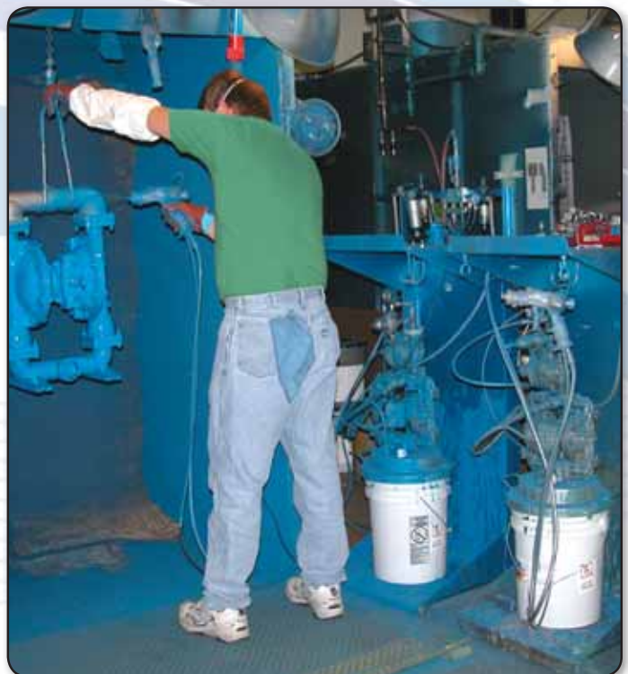
Pail mounted SANDPIPER® Pumps installed on paint spray booth station.
