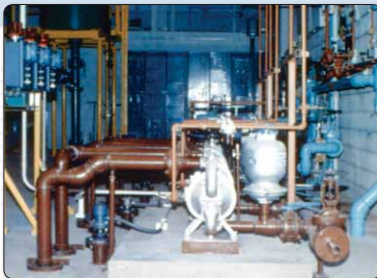
Heavy duty flap valve pumps with tranquilizers permanently installed in an automotive industrial waste treatment facility.
