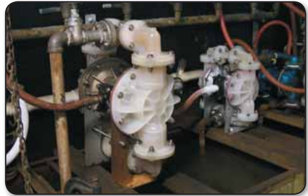
Standard duty polypropylene pumps installed for chemical processing.
