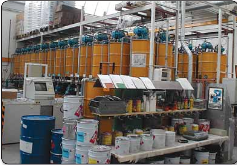
1" ball valve pumps installed in a paint mixing and tinting operation.
