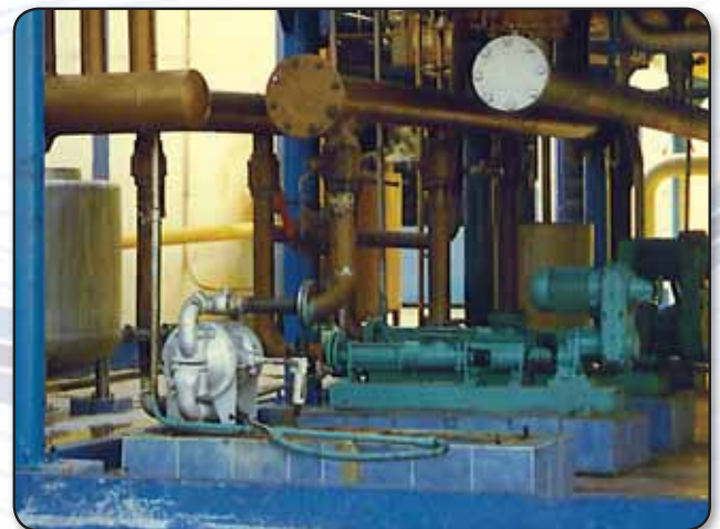
Solution providing AODD pump installation selected to reduce total costs of ownership and minimize floor space allocation.
