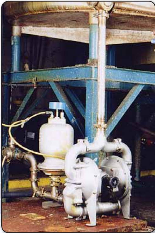
Heavy duty flap valve pump installed on an underflow sludge transfer application.
