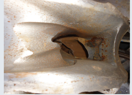
F6147A05 Impeller (standard) 2,145 hours inspection
