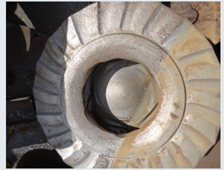
F6147A05 Impeller (standard) 2,145 hours inspection
